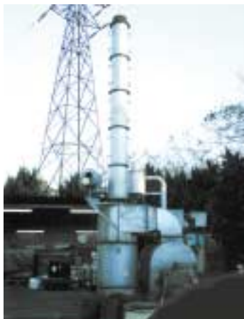
The Inctec Kansai plant: Prior to shutting down the incinerator
