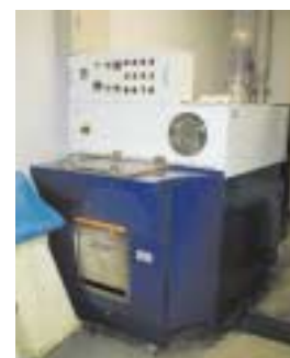
Food waste processing machine (located in the basement of the C&I headquarters)
