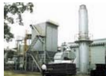
Dai Nippon Technopack Izumisaki plant: Incinerator
