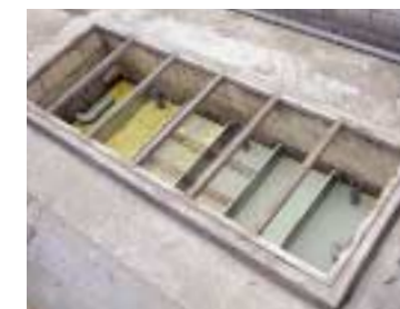
Dai Nippon Cup, Sayama plant: Oil-water separation compressor drain
